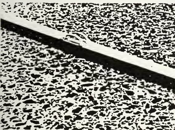
Fig. 3.2.1.6 — Wheel track wear
